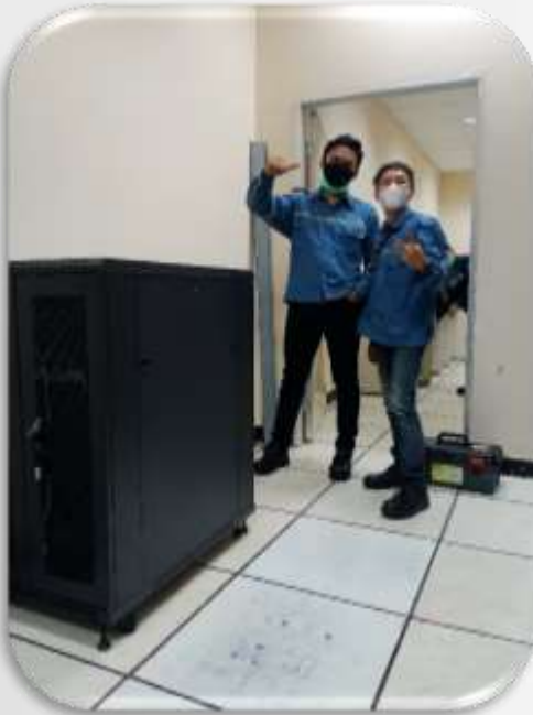
Isntalasi System DIS CEMS (Krakator Posco Energy)
