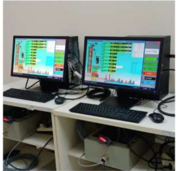
Isntalasi System DAS CEMS (Krakator Posco Energy)
